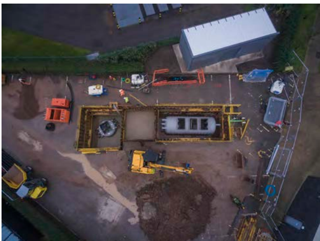
An aerial view of the new Energy Centre, WHR buffer tank, and valve chamber
